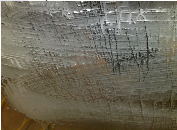
NOTE – Blade cut lines and protection damage
